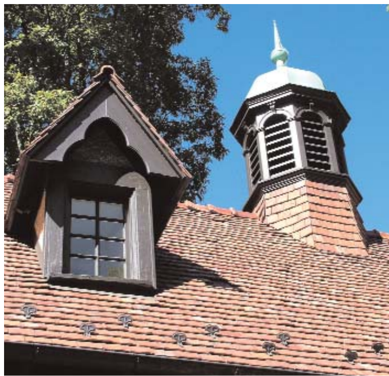
Two new dormers were added for extra light. They were designed to fit into the style without mimicking the originals. The cupola required extensive reconstruction – 25% of the woodwork was replaced and then painted to match what remained.
